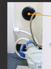
Generator room outlet
